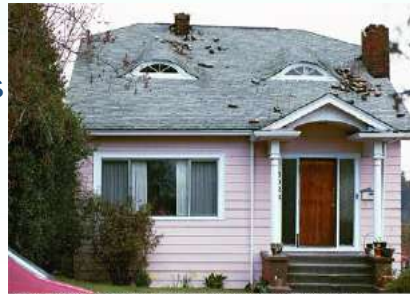
Seattle, WA, March 10, 2001 -- Chimney bricks crumbled during the earthquake.
